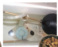
Building "B" is 5 years old and does not have a filter. Sediment and rust is seen in toilet tank and tap aerator.
