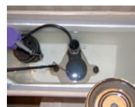
Building "A" is 7 years old and had a JUDO PROFIMAT water filter installed when constructed. Sediment and rust free toilet tank and tap aerator.
