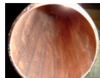
3" Copper Pipe - The way it should look!
